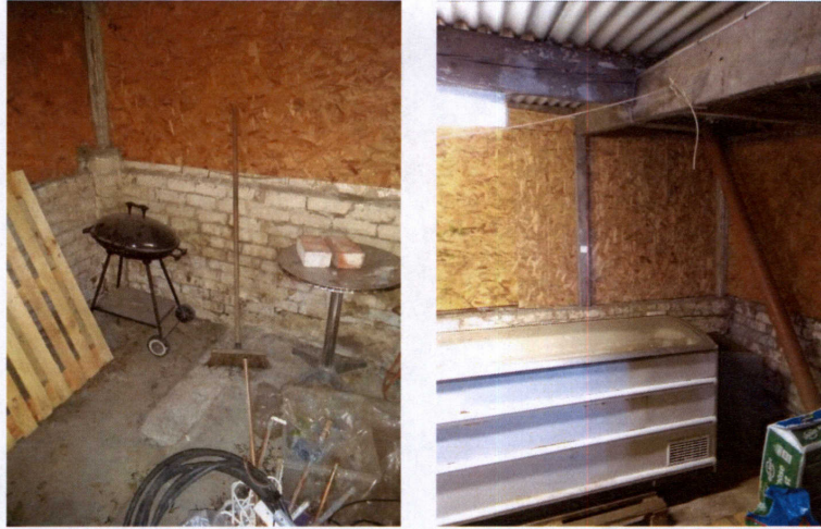
Images 05 / 06 - Internal view of store building looking towards boundary wall showing brick and OSB construction.
